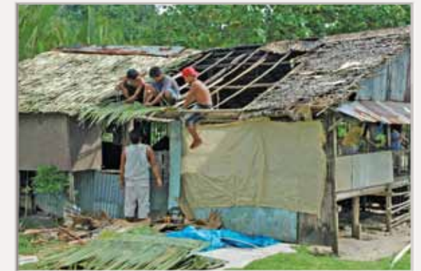
Working together to make a new thatch roof (photo from Walung, Kosrae State)
